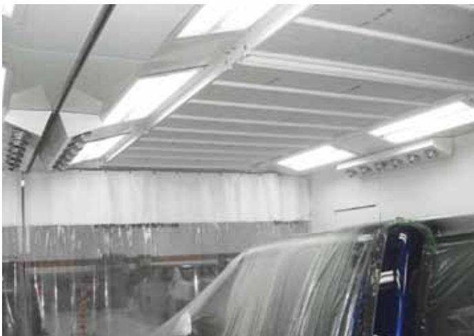
Drive-thru prep station with four horizontal modules
